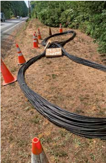
Crews installing Peninsul School District's new fiber optic cable marked everything "Not Copper" to prevent theft. Tim Heitzman, KP News
